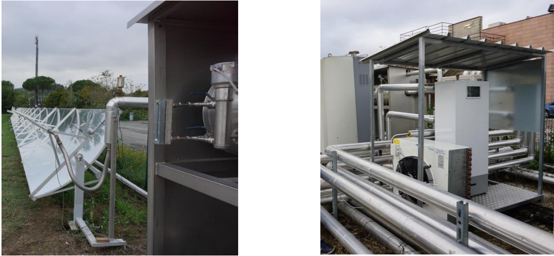
Fig 6 The solar powered ORC. Left: the collectors; right: the ORC prototype and the dry cooler
